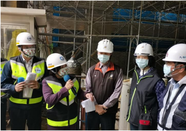
Picture 1: Minister Hsu Ming-chun led a labor inspection team on a spot inspection tour and declared 2021 as the “Year of Strengthening Prevention of Occupational Disasters in the Construction Industry.”
